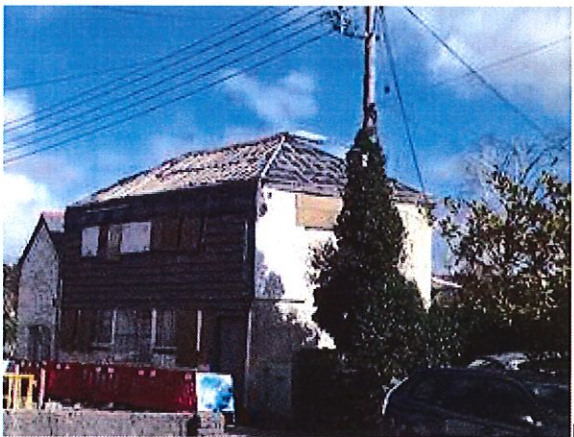
The sorry state of St Day Carpenter's Shop
